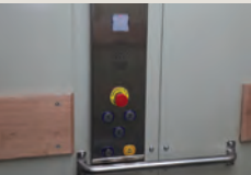
Lift car operating panel with autodialer and display
