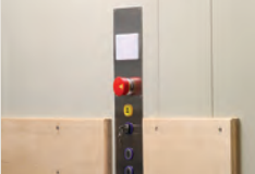
Lift car operating panel
